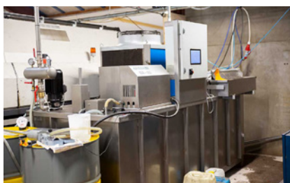
The central filtration system for filtering the lubricant.
